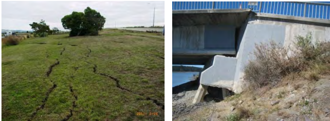
Figure 18. Liquefaction-induced damage to South Brighton Bridge.
