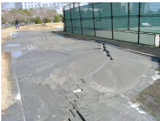
Fig. 14 Liquefaction in Urayasu City of Chiba
