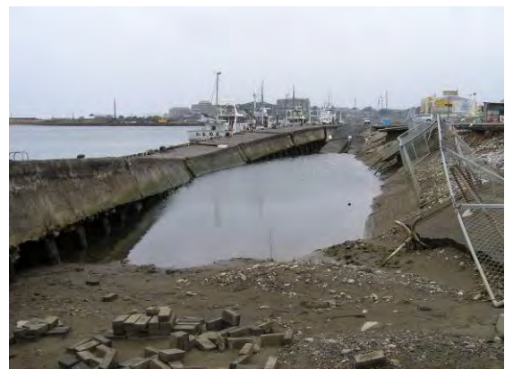
Fig. 20 Damaged quay wall in Nakaminato Harbor
