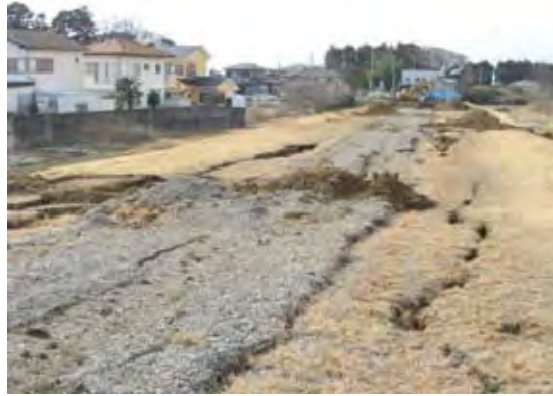
Fig. 25 Liquefaction-induced lateral spread of Naka River levee
