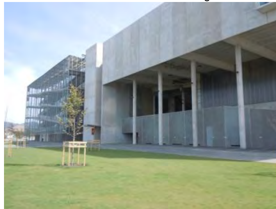
Figure 12. Liquefaction adjacent to AMI stadium.
