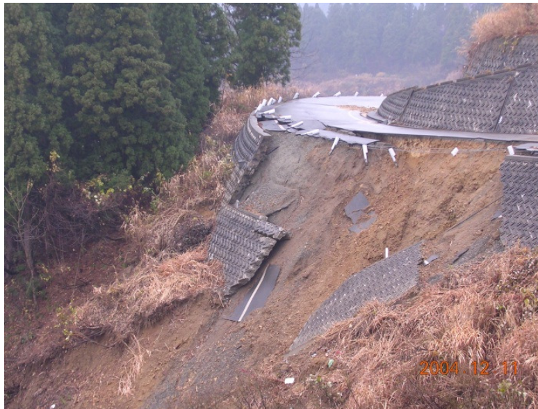
Fig. 22 Retaining wall sliding down with road embankment.
